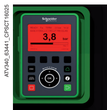
Detected fault: The red screen backlight is activated automatically
